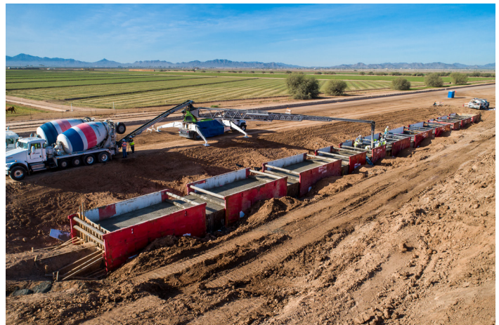
Achen-Gardner crews used trench boxes as the framework for the concrete encasement on our Ak-Chin Link Pipeline Repair and Mitigation project.
