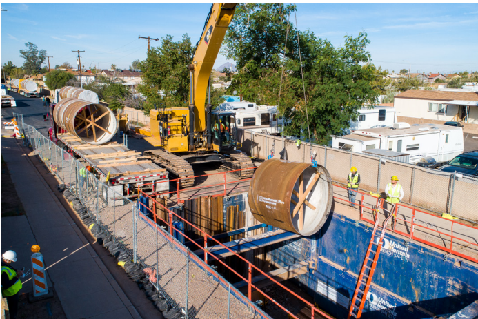
Installation of welded steel liner east of Mesa Drive on our Val Vista Transmission Main Rehabilitation CMAR project.
